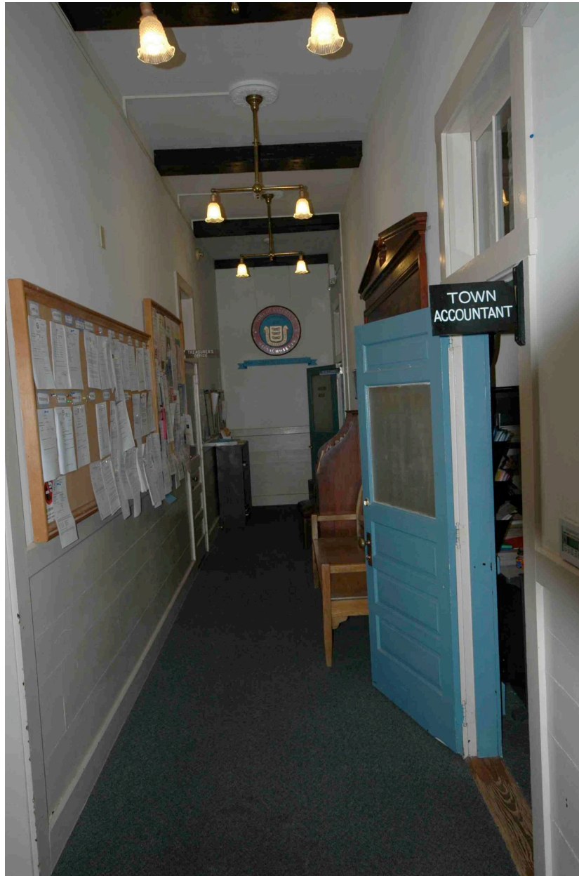
Main Corridor Blocked by Vault Addition
