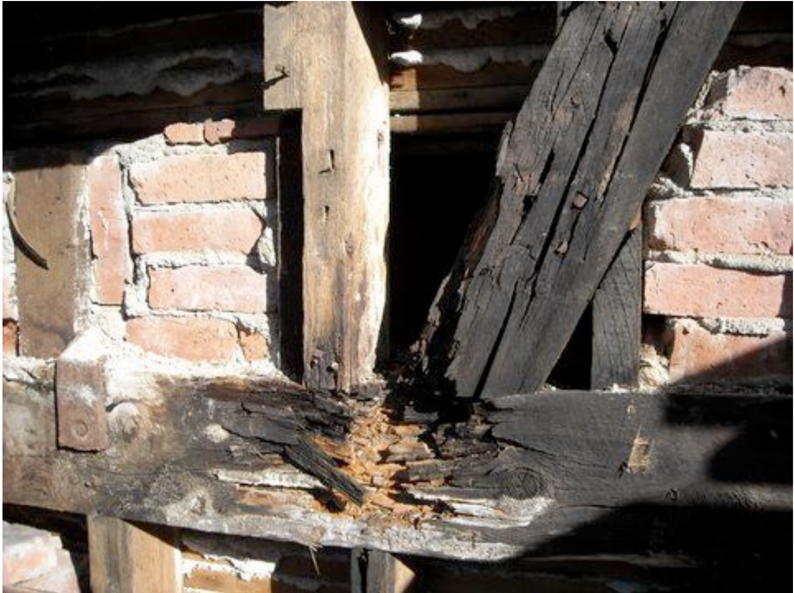
Deteriorated Structural Framing
