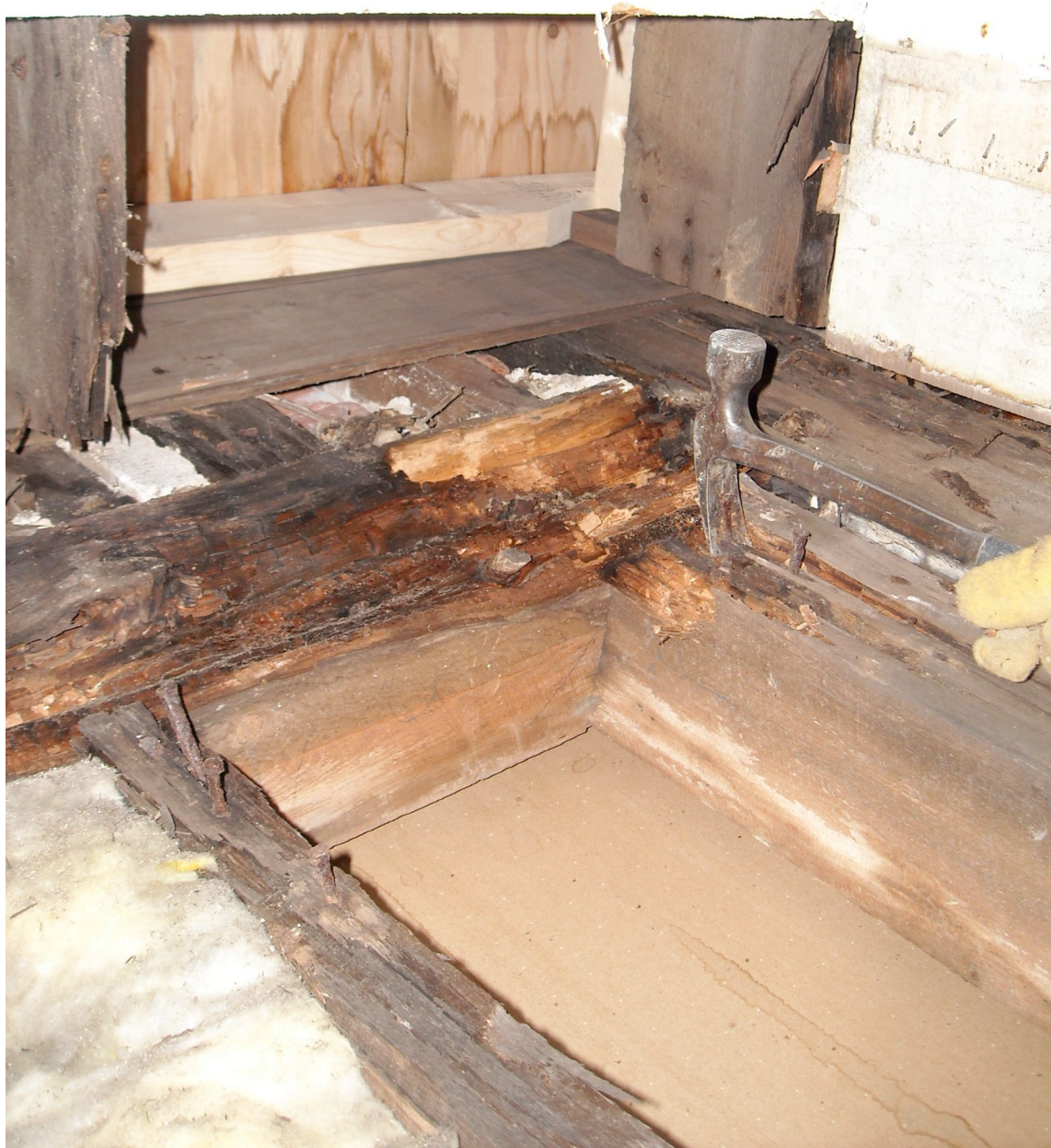
Additional Structural Deterioration
