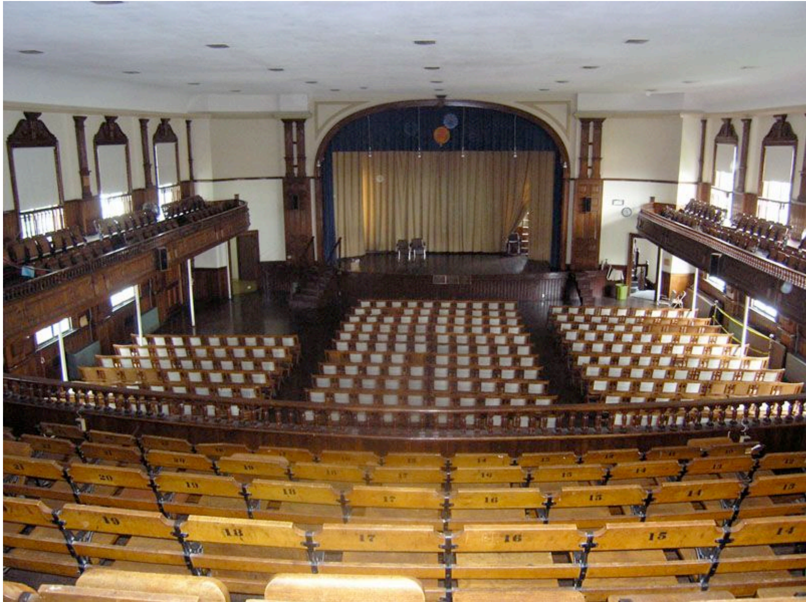
Pre-Restoration View of Auditorium Looking Toward Stage Showing Flat ca.1950 Ceiling without Chandelier
