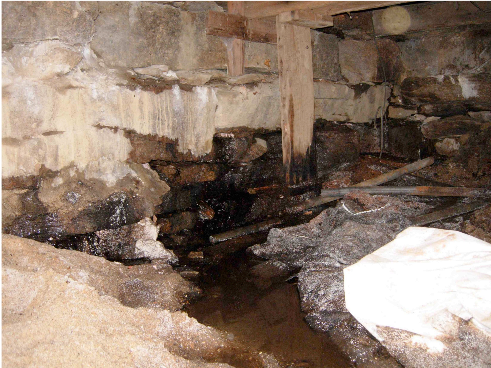
Water Ran across Basement Dirt Floor into a Culvert and into the Adjoining Stream
