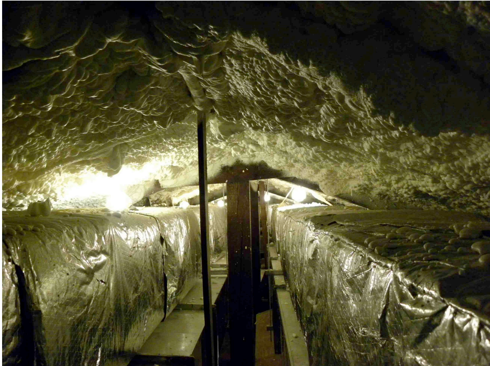
R-38 Ceiling Insulation with Oversized Ductwork to Provide Quiet Ventilation to the Auditorium and Free Cooling During Spring and Fall Temperatures
