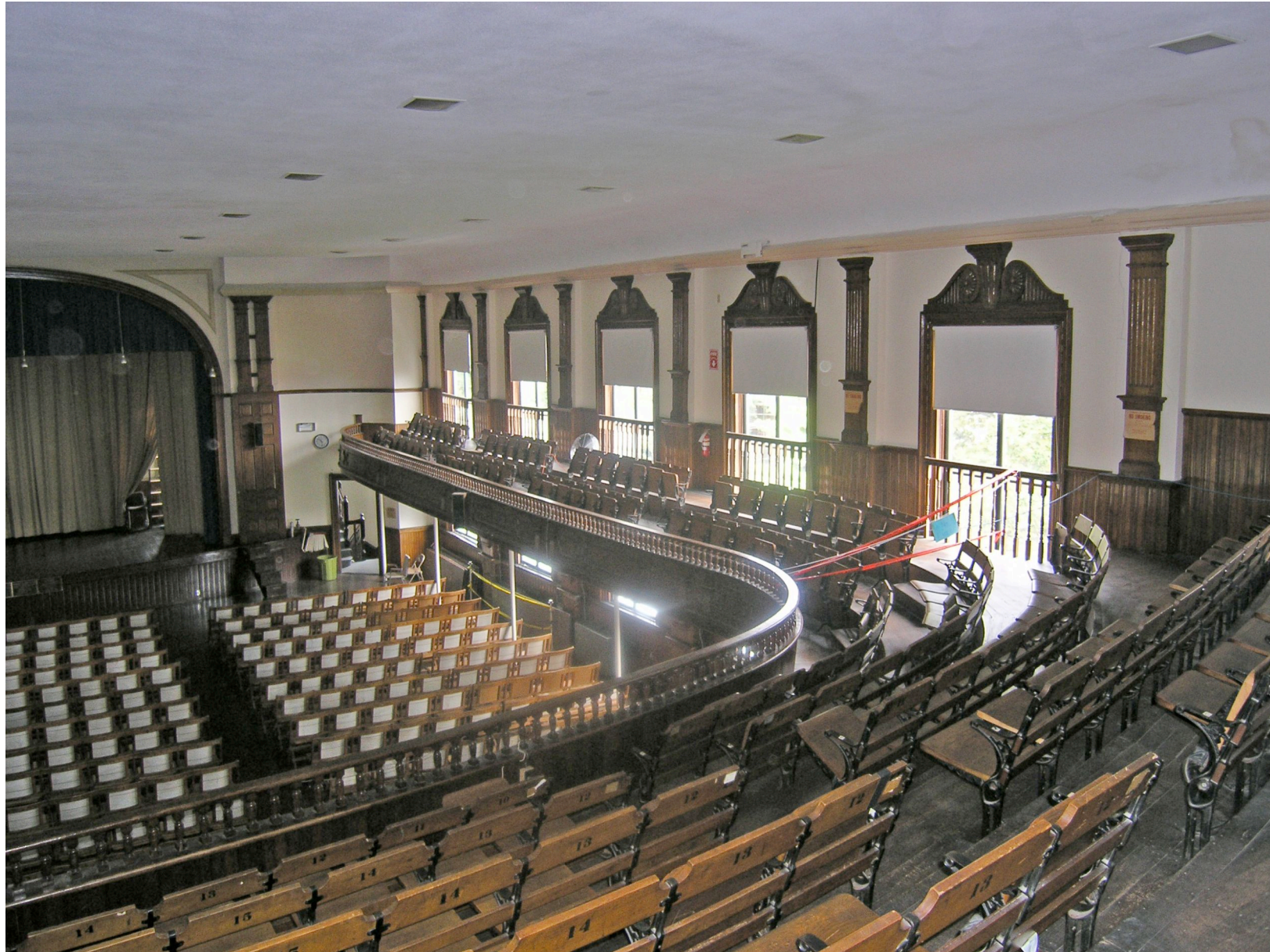
2008 View of Auditorium from Balcony. Side balconies were closed even before structural assessment was undertaken, due to excessive vibration.
