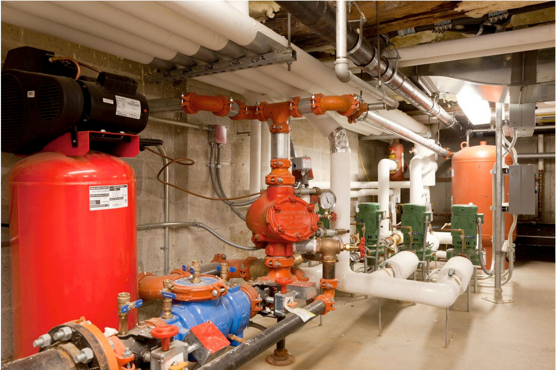
New High Efficiency Heating Equipment
