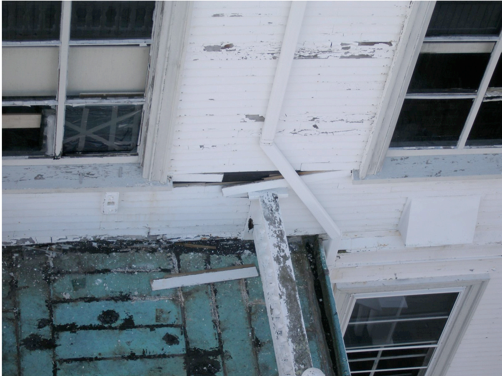
Closeup View of Deteriorated Siding, Windows, Roofing and Balustrade
