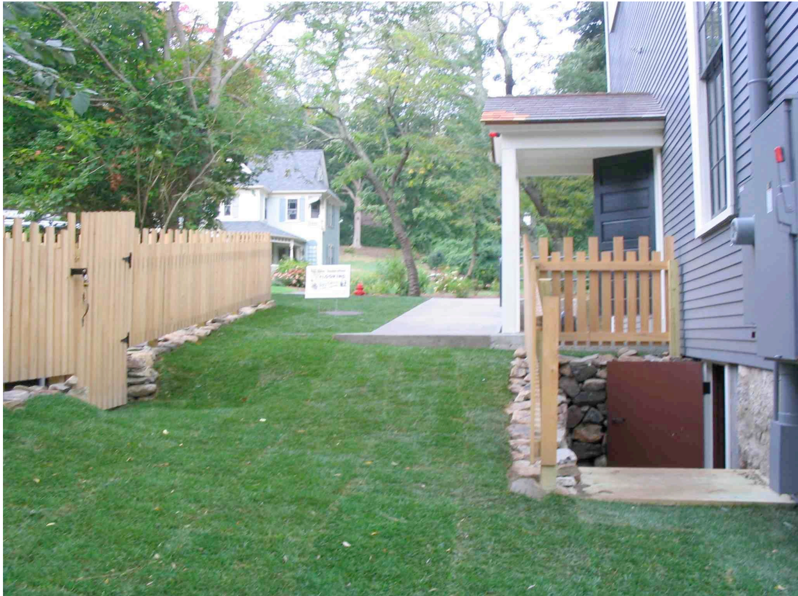
Rear of Town Hall with Entrance to Mechanical Equipment Area at Right, and Fence around Gas Chillers at Left
