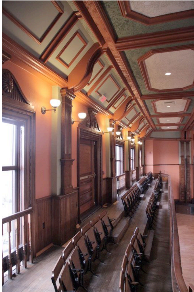
Restored Balcony Side Wall with Replica Energy Efficient Wall Sconces and Coffered Ceiling
