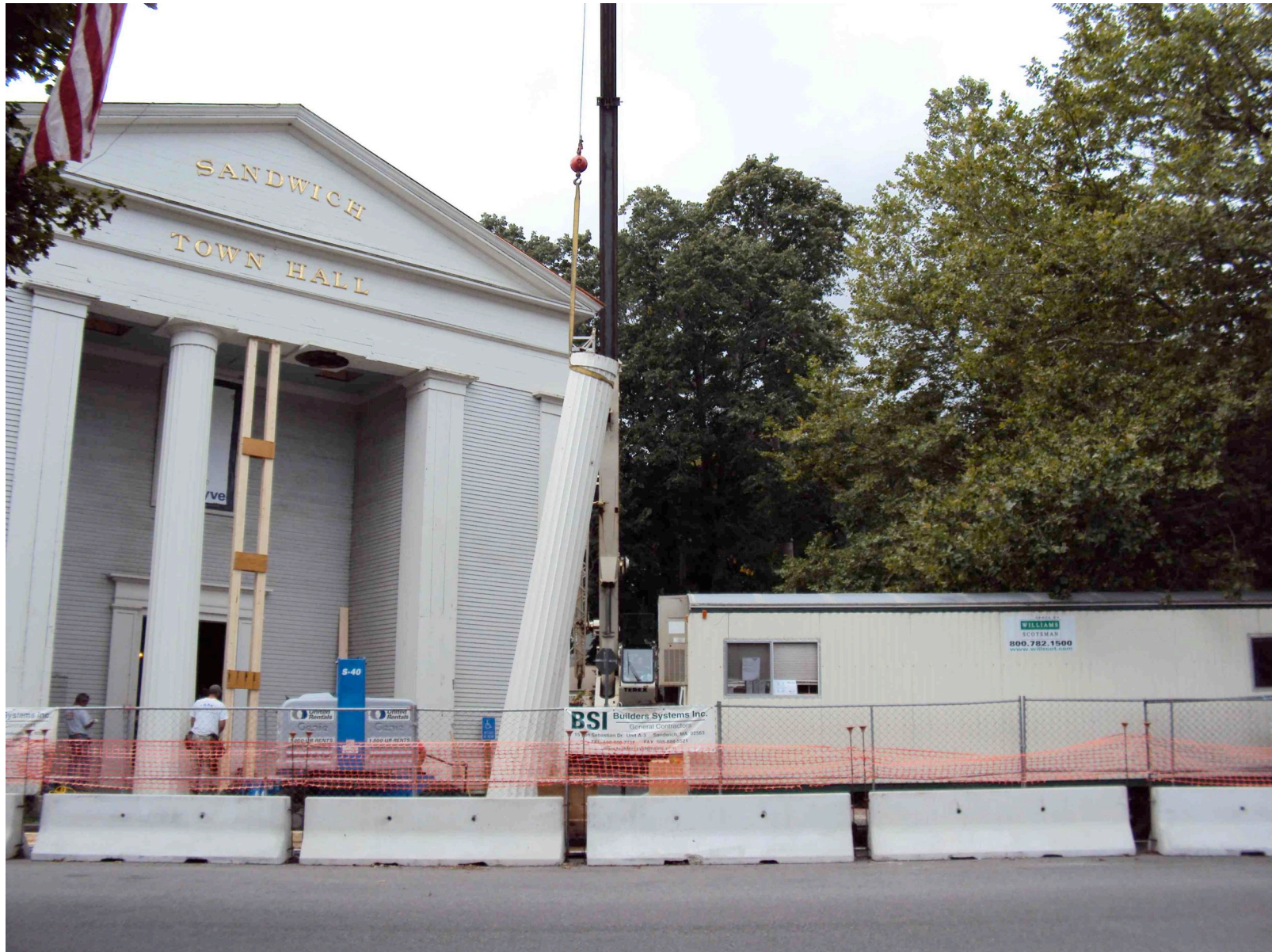
Restoration and Renovation Work Included Removal of Columns so the Entry could be Raised 7" to Provide an Accessible Front Entry
