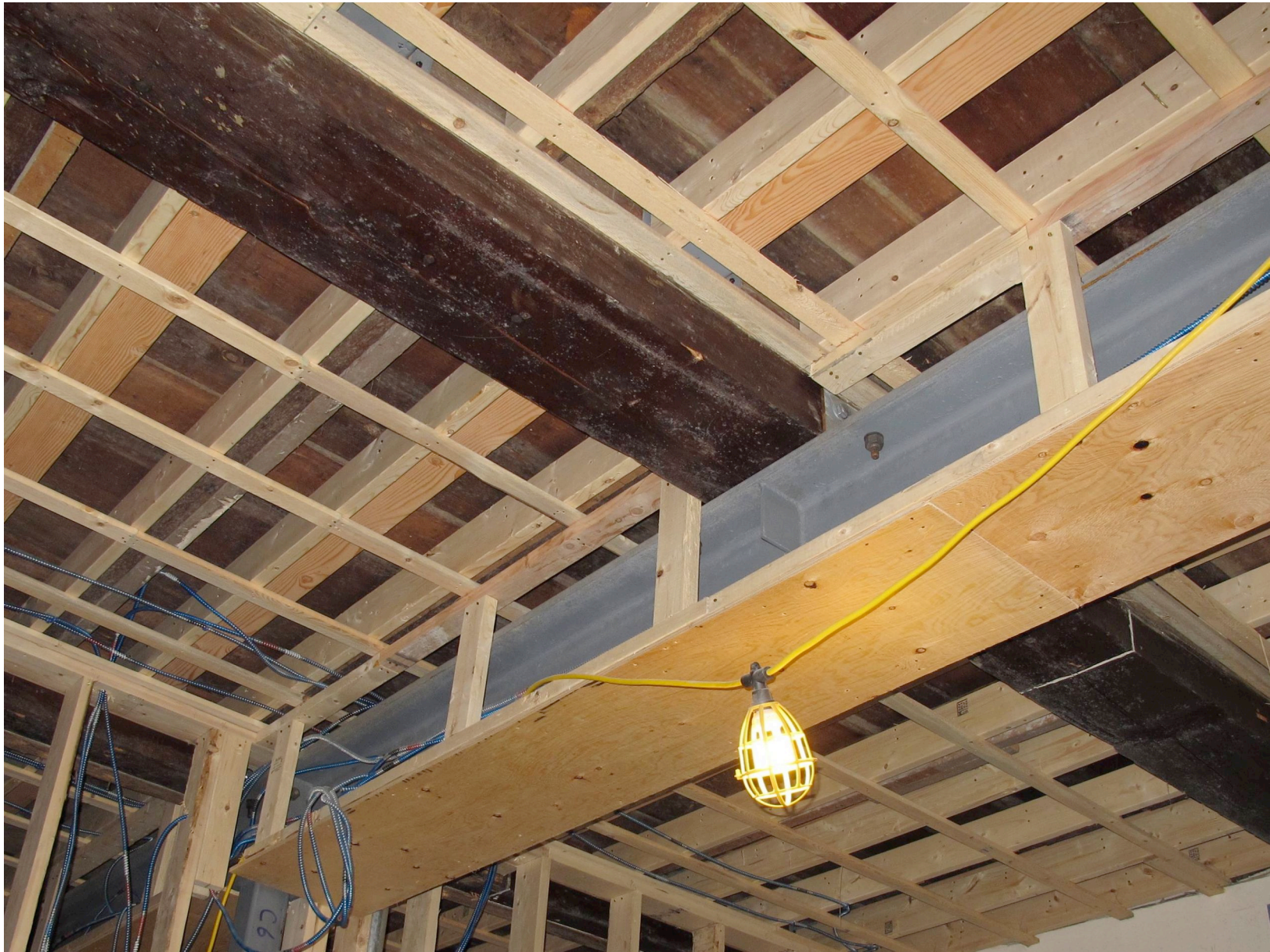
New Steel Summer Beams were Added to Provide Adequate Second Floor Capacity
