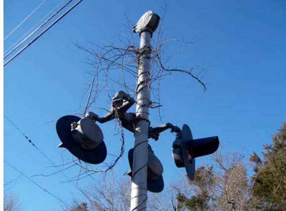
Figure 2.5-25: A Crossing Signal at Old Dock Road Overgrown With Vegetation
